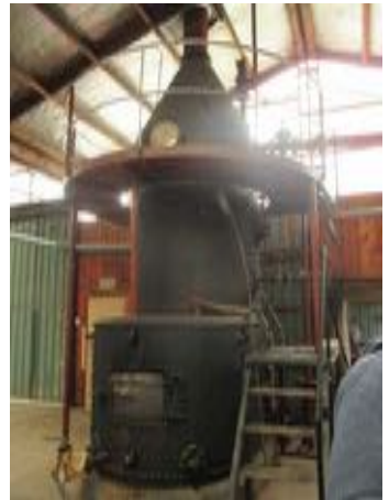
Gladstone big boiler.
