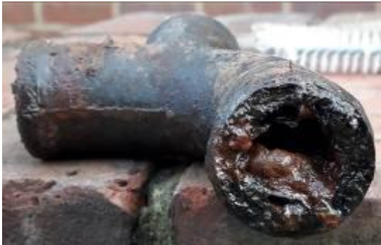
Photo 1 – Sludge in heater elbow
